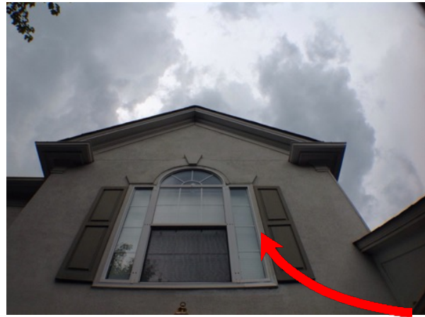
Walls/Siding/Trim - Cracking trim above window.
