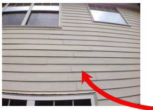
Rear Exterior Walls/Siding/Trim Caulked joints of siding are cracking.
