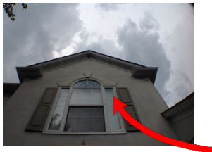
Front Exterior Walls/Siding/Trim Cracking trim above window.
