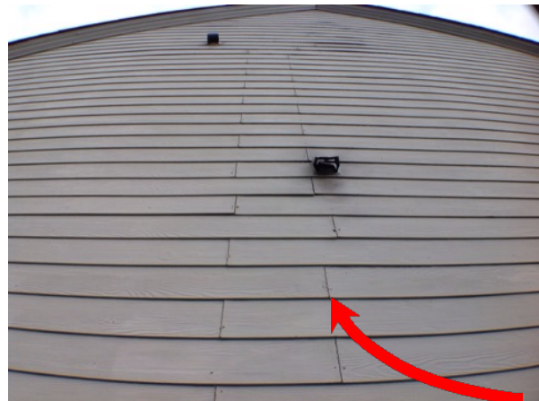
Walls/Siding/Trim - Caulked joints of siding are cracking.
