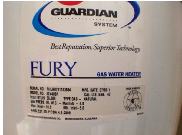
Water Heater - MFG Date
