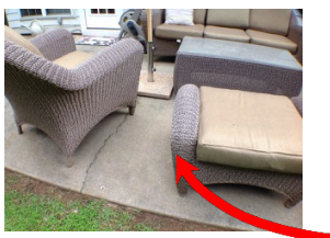
Rear Exterior Patio/Porch Crack up the middle.
