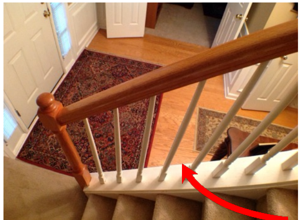
Banister - Banister is loose.
