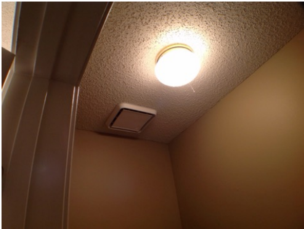
Exhaust Fan - In commode room.
