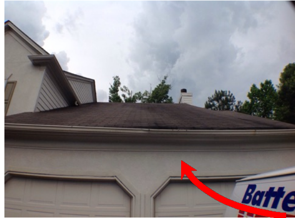
Roof/Trim - Bent Gutter
