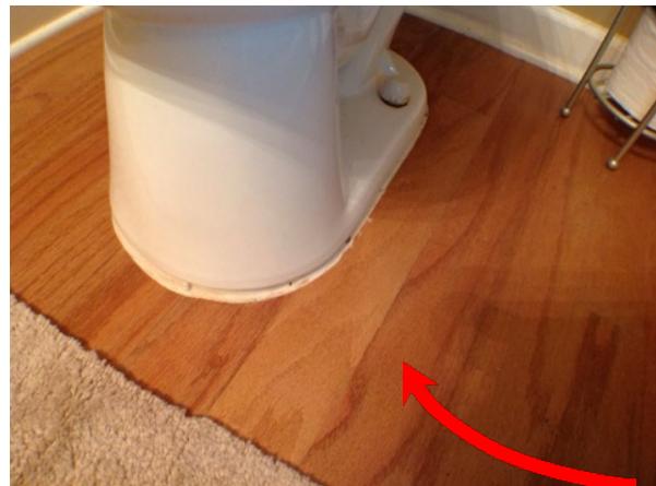
Commode - Discolored and cracking caulk.
