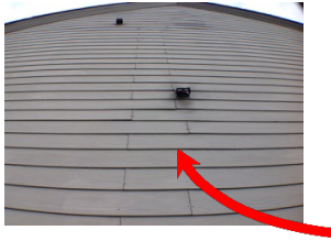
Front Exterior Walls/Siding/Trim Caulked joints of siding are cracking.
