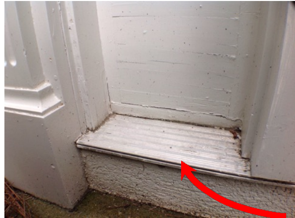
Front Door Exterior - Slight cracking of trim caulk and paint.
