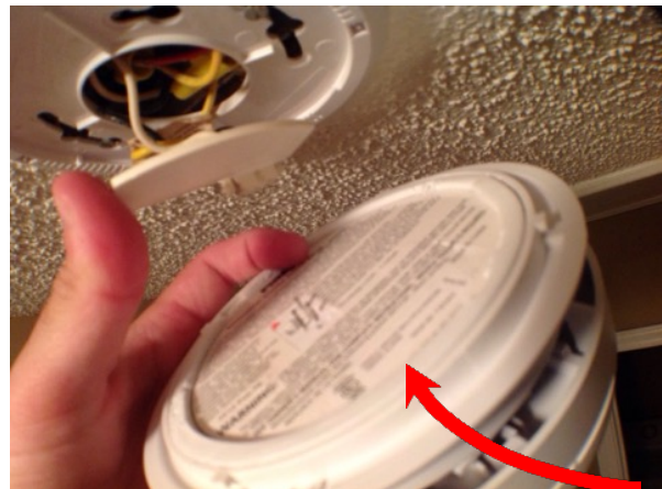
Smoke Alarm - Wrong connection for alarm, but still works.
