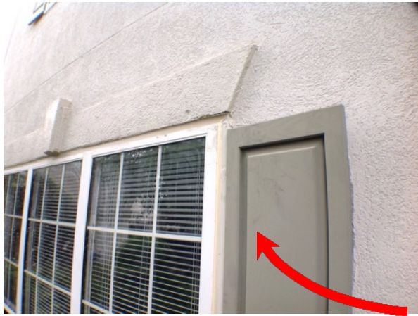
Walls/Siding/Trim - Discolored trim and caulk.
