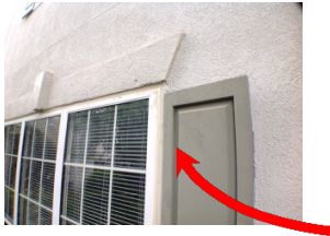
Front Exterior Walls/Siding/Trim Discolored trim and caulk.
