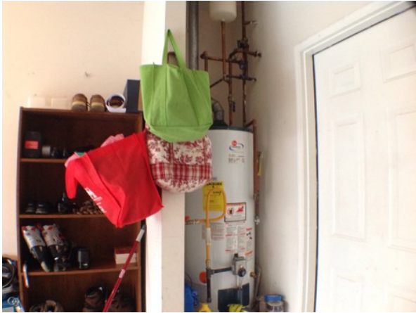
Water Heater - Rheem Gas
