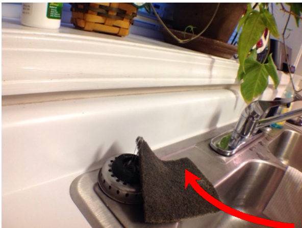
Counter Top/Back Splash - Caulk discolored and cracking behind the sink.
