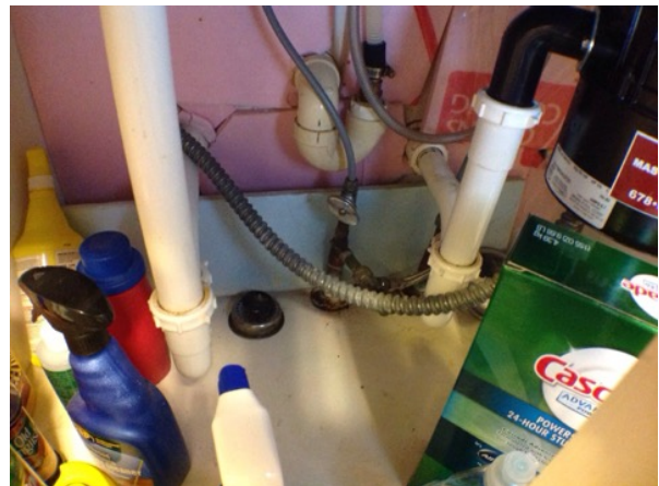
Cabinet Under Sink
