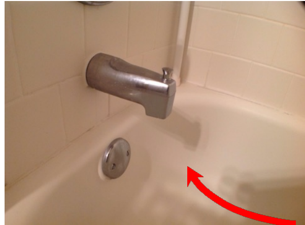
Tub/Fixture - Caulk is slightly Discolored.
