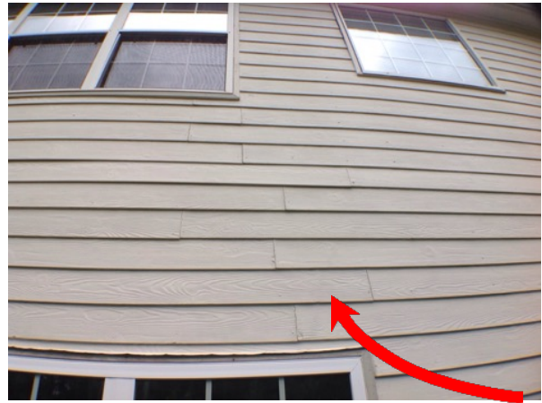
Walls/Siding/Trim - Caulked joints of siding are cracking.
