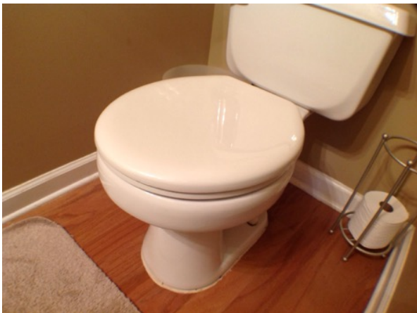
Commode - Caulk at floor is discolored.
