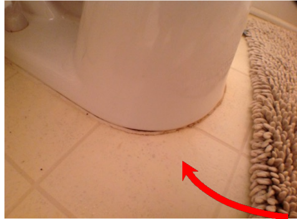
Commode - Discolored caulk and slightly pulling away.
