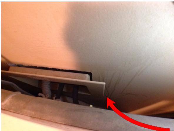
Walls/Paint - Moisture streaks on back wall.
