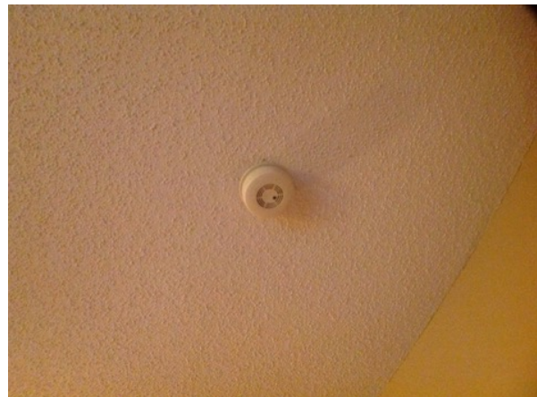
Smoke Alarm - Out of date and failed to test properly.
