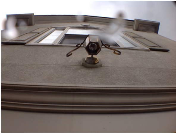
Light Fixtures - Does not turn on.
