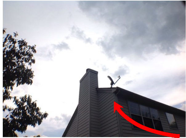
Walls/Siding/Trim - Where the chimney trim meets the roof, it (trim) is chipping.
