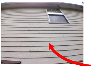
Rear Exterior Walls/Siding/Trim Caulked joints of the siding are cracking.
