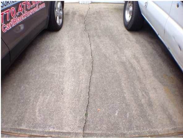
Driveway - Center Crack
