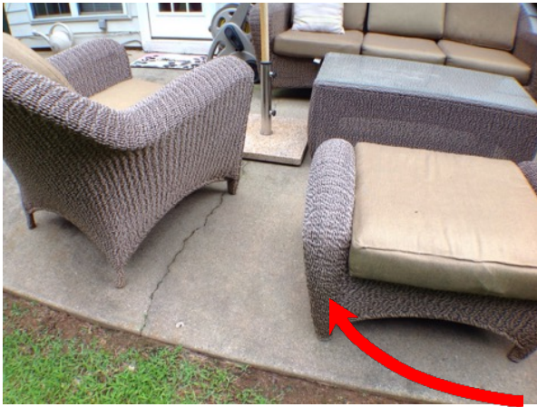
Patio/Porch - Crack up the middle.
