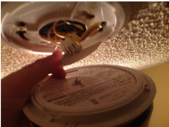
Smoke Alarm - Wrong connection, but still functions.
